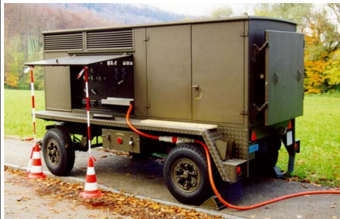
Fig. 8: 120 kW Diesel power generator, driving the "large" shakers shown in Figures 5 and 6.
