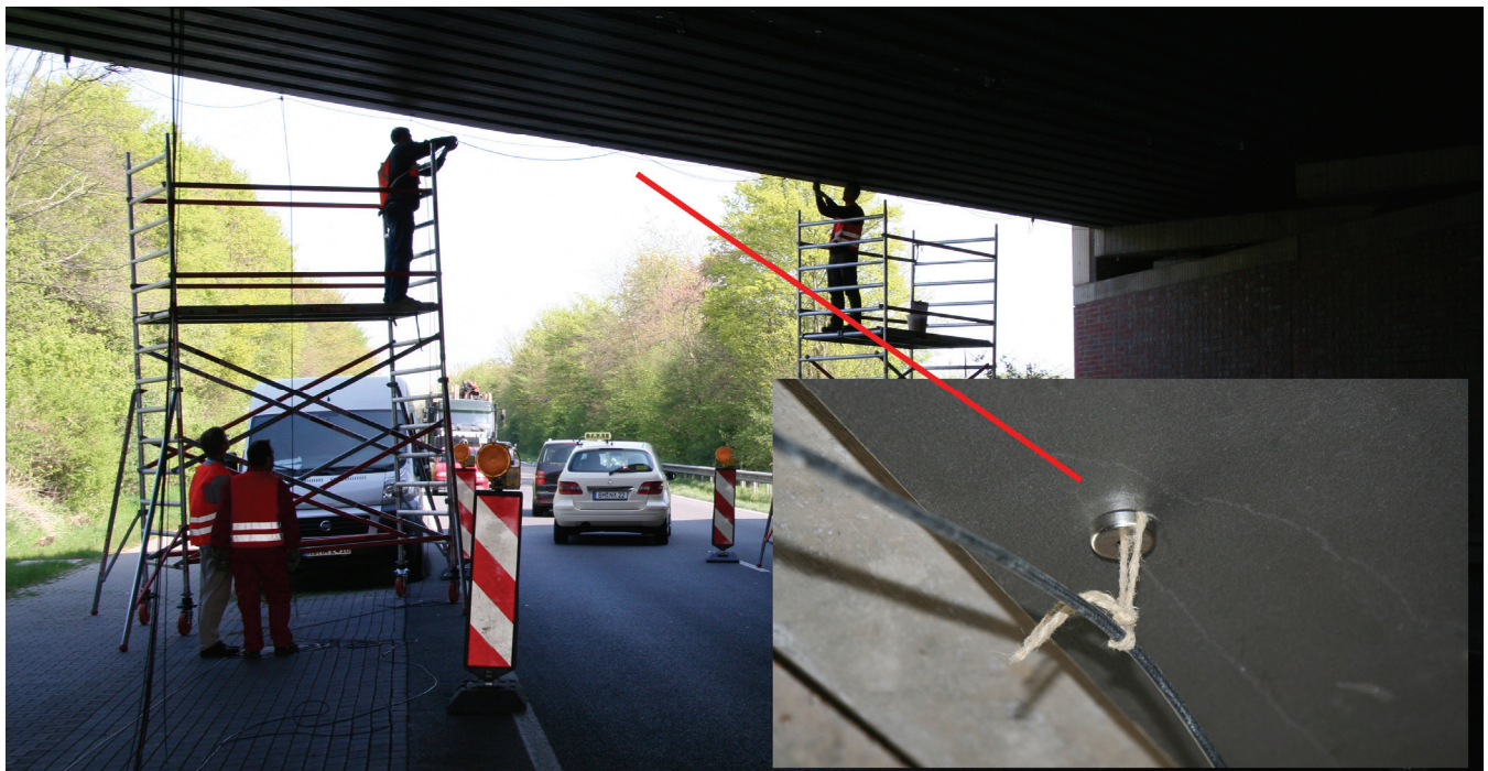
Fig. 10: View underneath the Erfttal Bridge on measurement day 2. View direction reverse to the one in Figure 9.
