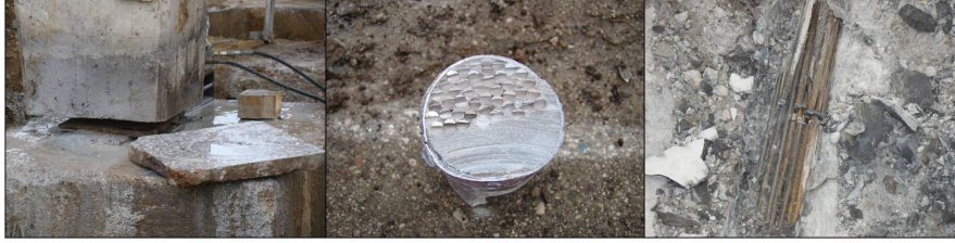
Fig. 3 Destructive damaging; a) cutting through one of the columns, b) and c) successive intersecting of prestressing tendons [10].
